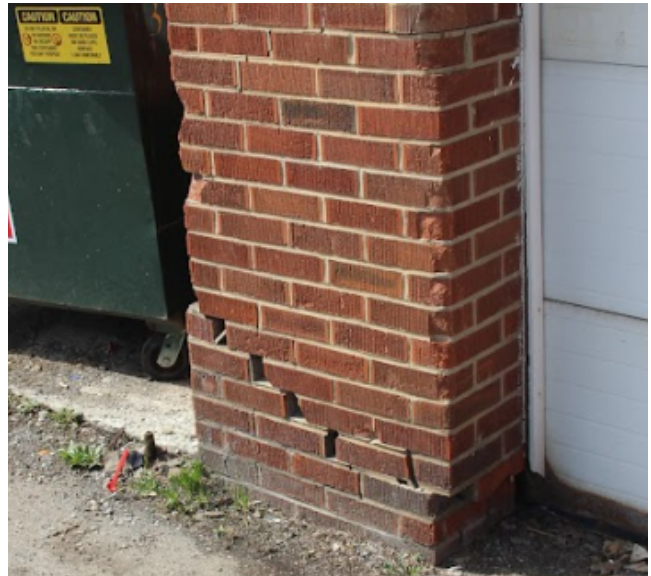
Structural damage is noted at the Police Garage.
