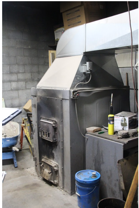
Wood-Burning Furnace in Public Works Facility
